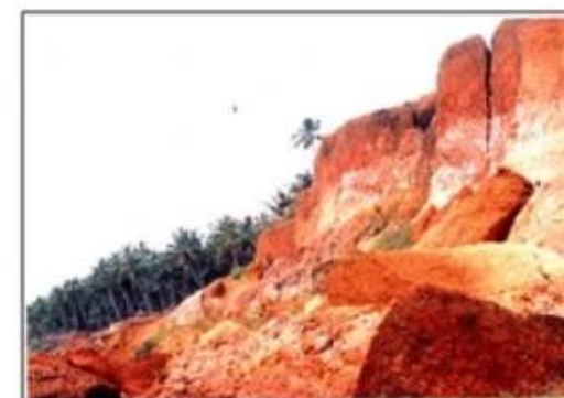
Toppling failure at Varkala.
